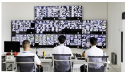
Campus security and logistics control room — 82,000 m 2 site
